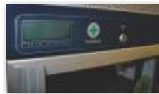
Large Control Panel
